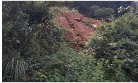
Fig. 1. Slope in Kanjikuzhi
