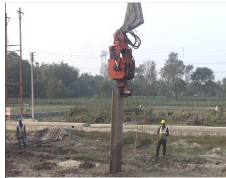
Photograph 2: The driving and withdrawal of Section of Steel Sheet Pile with Vibro-hammer by placing it at top of Sheet Pile (Courtesy: M/s. L&T Construction, Transportation Infrastructure)
