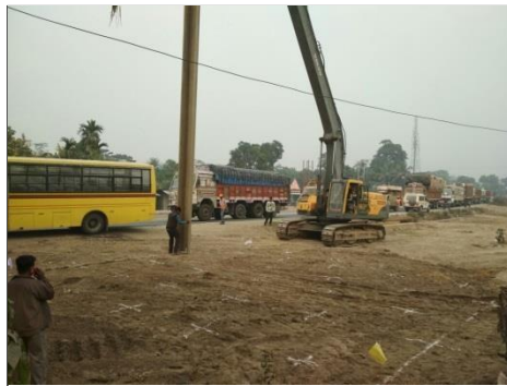
Photograph 1: Ground Treatment by Vibro-probing with Section of Steel Sheet Pile at the marked grid points covering Foundation Base and its beyond area (Courtesy: M/s. L&T Construction, Transportation Infrastructure )
