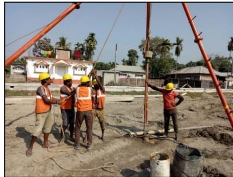
Photograph 3: Showing Field SPT in progress at the foundation base area of substructure after “Vibro-probing” method of densification (Courtesy: M/s. L&T Construction, Transportation Infrastructure )
