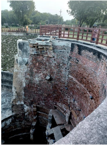
Fig. 9 Deterioration of the wall (Section 2)
