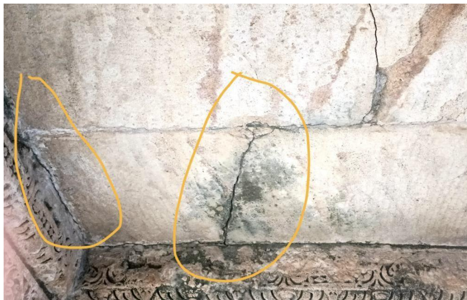
Fig. 8 Moderate cracks in the ceiling (Section 3)
