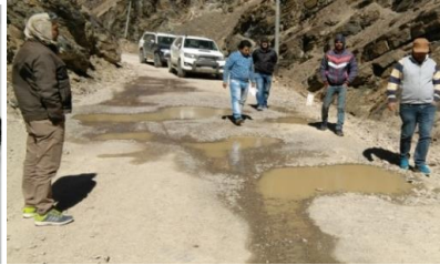
Fig.5. Seepage water visible on CRM surface before installation
