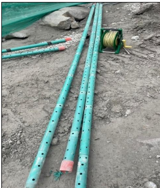
Fig. 3a. Perforated Pipes for Observation Bore Hole
