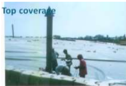
Fig. 12. Top coverage and gas vent
