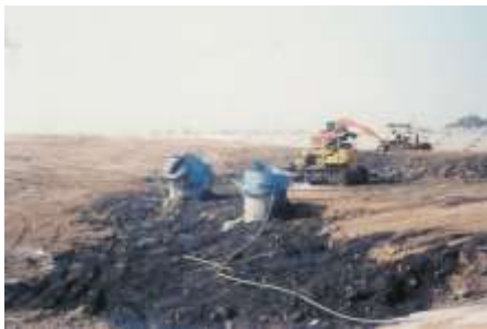
Fig. 17. Leachate collection wells
