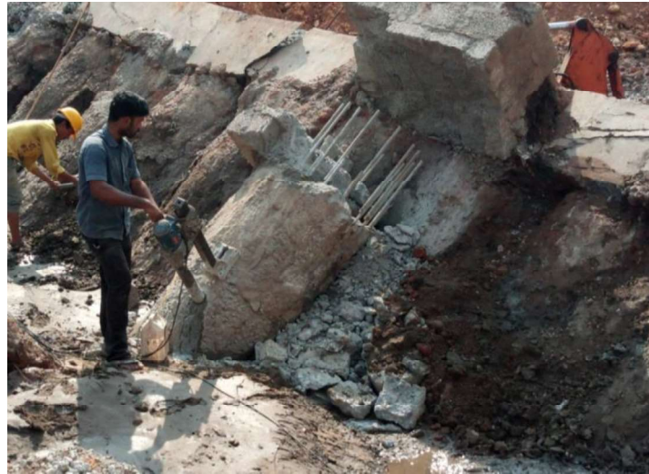
Fig. 7 (a). Extracting core from failed pile at site
