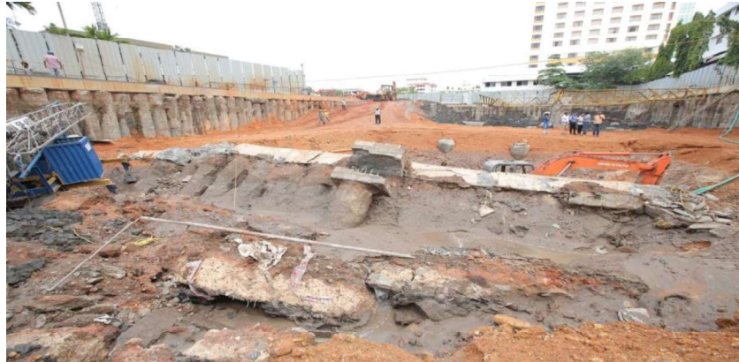
Fig. 4 (b). Photo of collapsed touch pile system at Kaloor, Cochin
