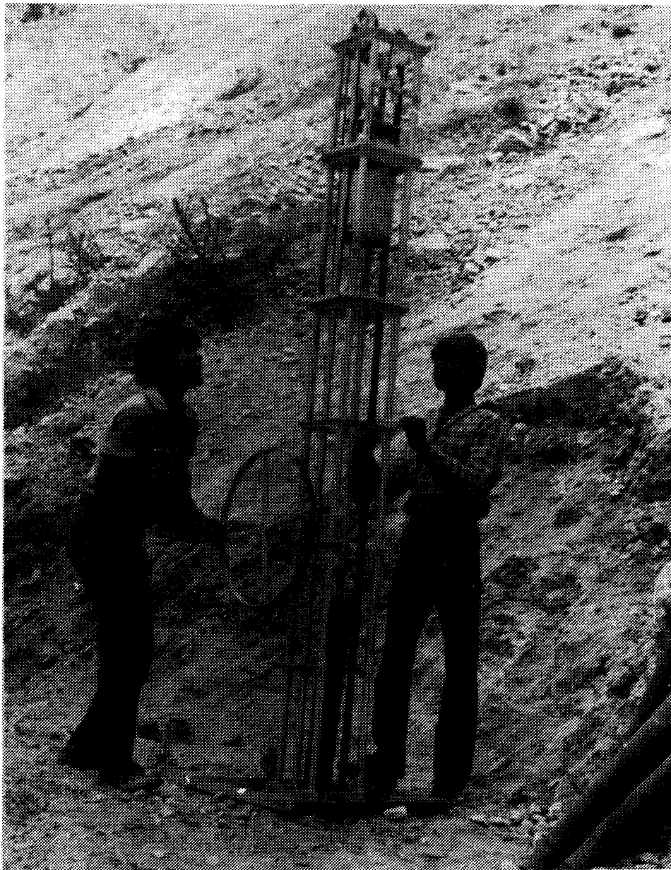
Figure 27 Stitching of colluvium on the slope at Kaliasaur by a simple Lowcost Timber piling Machine
